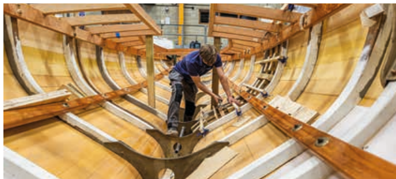
W-8 RIPPLE (ex-DINAH) currently being completely restored (reconstructed frame by frame) at Berthon, teaching apprentices tradition as well as modern skills © Harry Shutler, Berthon
